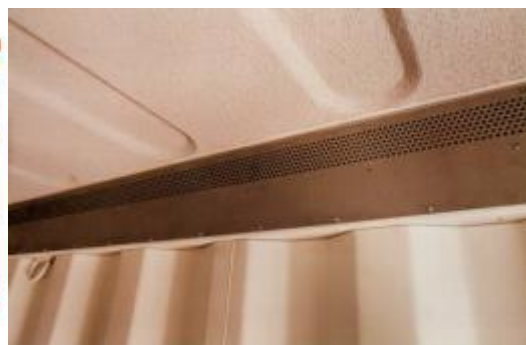
Figure 3.18 – Ventilating container inner grill
